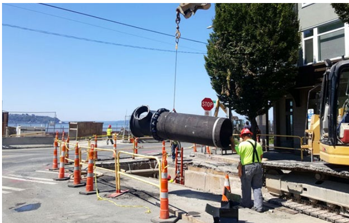
The last piece of stormwater infrastructure was installed at the jack and bore pit on Pine Street.
