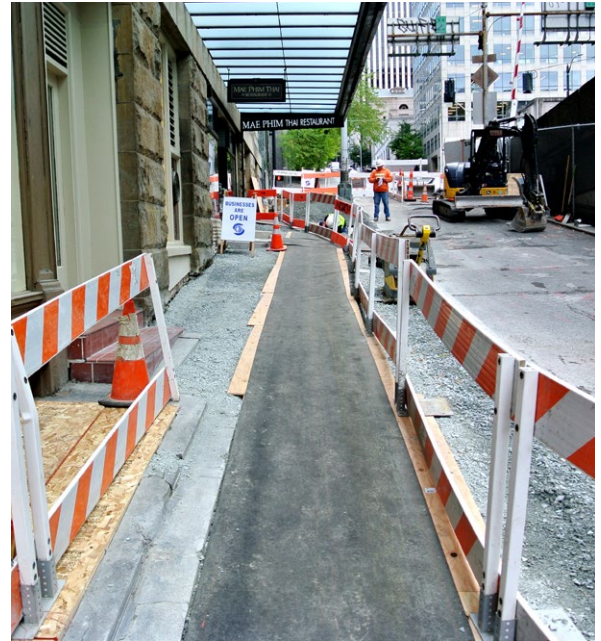
The sidewalk along Columbia Street was demolished and regraded ahead of the new concrete sidewalk build.
