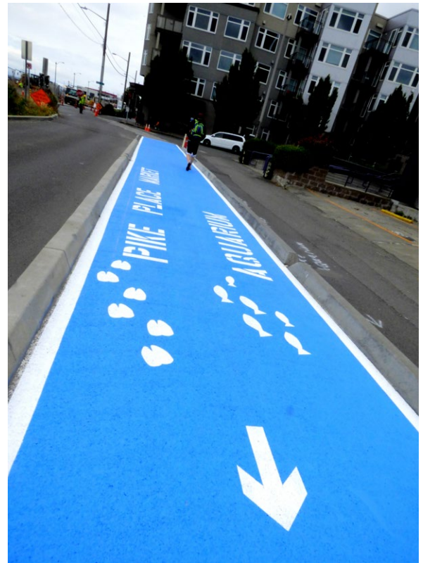
The newly repainted multi-use path on Alaskan Way helps users navigate the waterfront during construction.
