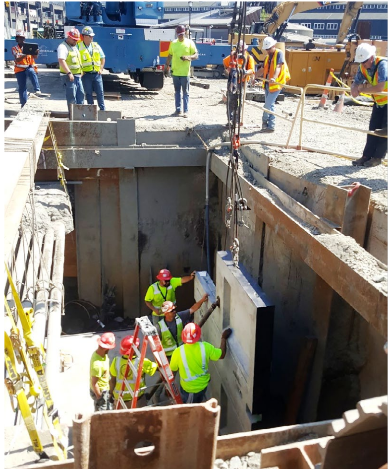
Crews installed the wall of a new vault as part of utilities relocation work.
