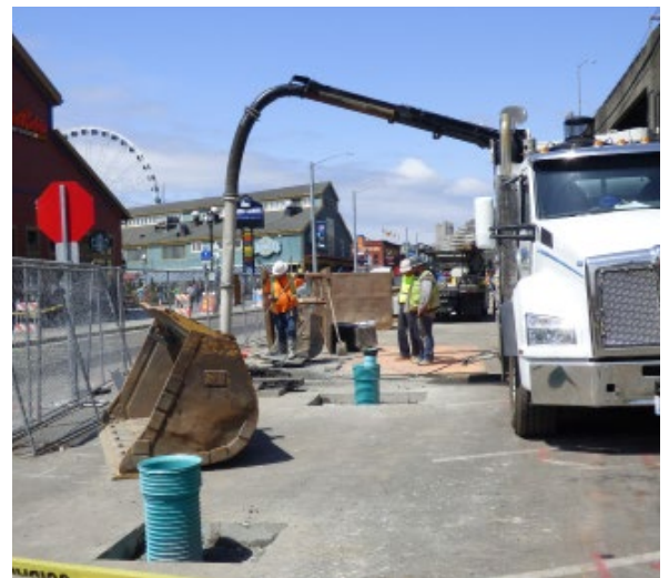
Crews used a site vacuum truck to search for and expose existing underground utilities.
